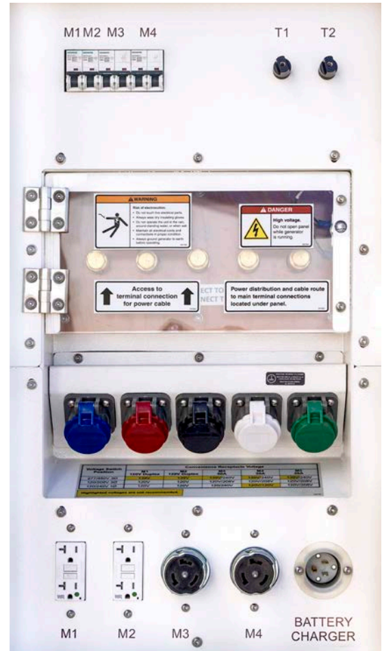
Convenience receptacles, weathertight camlock connections
